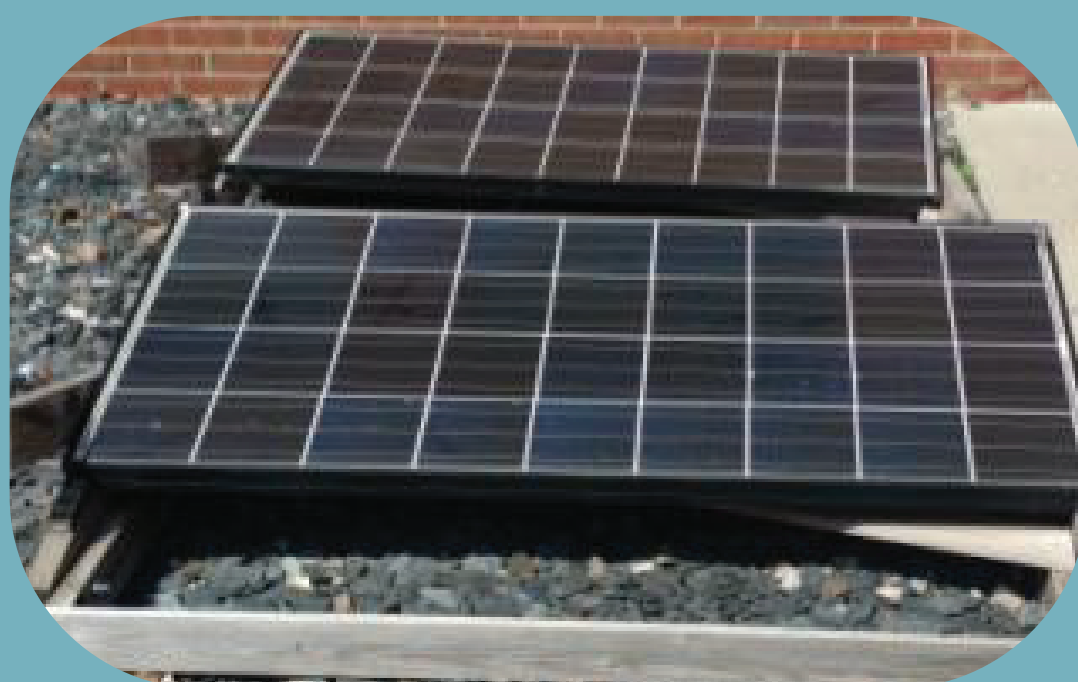
Solar Panels in Coover
